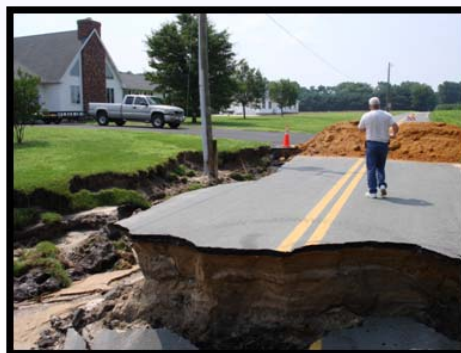
An entire section of Indiantown Road washed away in Dorchester County as a result of flooding in 2006.
