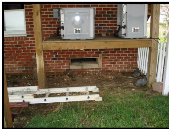
A homeowner elevates critical HVAC components for their home, mitigating flood damage
