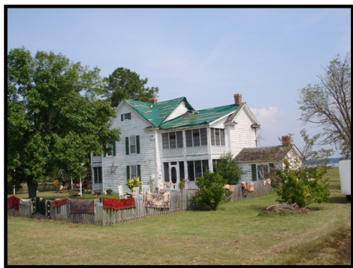
A home in Southern Maryland that received significant roof damage and flooding during Tropical Storm Ernesto
